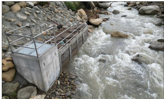
Figure 4: San Antonio Creek Diversion Structure (January 15, 2023) Source: Report of Operations – January 2023 San Antonio Creek Spreading Grounds Project Pilot Diversion Test, prepared by Rincon Consultants, Inc. (February 21, 2023)
